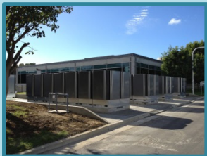
Top: Plug Power fuel cell system at a CSX site.
