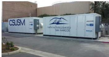
440-kW Doosan Fuel Cell America system at California State University, San Marcos (CSUSM).
