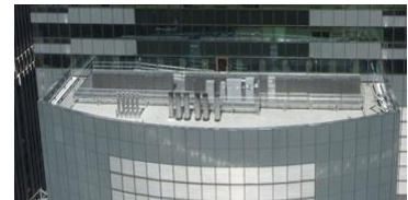
750-kW Bloom Energy rooftop installation at Morgan Stanley’s global headquarters in New York City.
