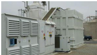
1.4-MW FuelCell Energy fuel cell power plant at a water quality control plant in Riverside, California.
